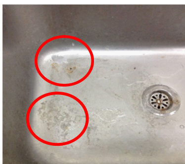
Fig. 4: A sink with spots of corrosion (red circles)
