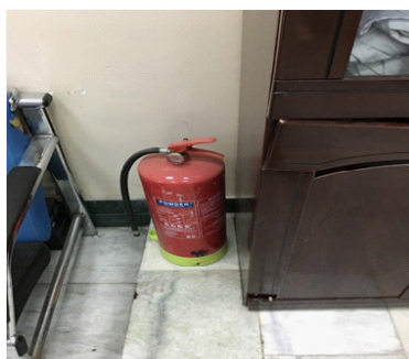
Fig. 7: An extinguisher located in a hidden place
