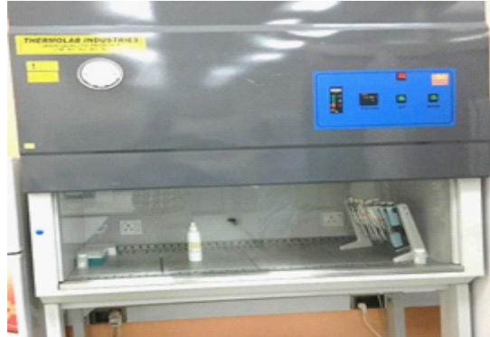
Fig. 12: A new biological cabinet installed in the renovated laboratory
