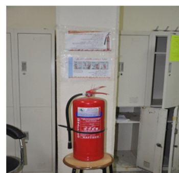
Fig. 7: A fire extinguisher improperly placed on a stool
