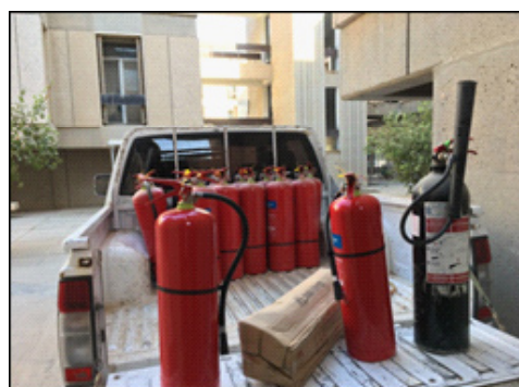
Picture 5: Purchasing new dry powder extinguishers
