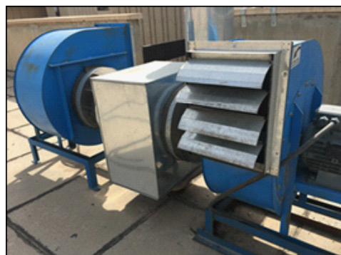
Picture 3: New ventilation systems
