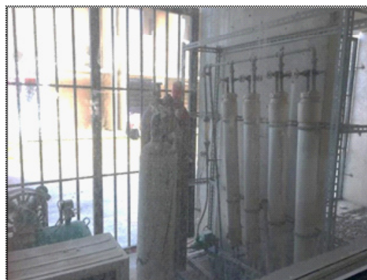
Fig. 5: Gas cylinders in a safe place
